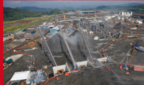
Each of the main crusher's three production lines has sufficient installed capacity for crushing 1,100 tons of basalt per hour.
