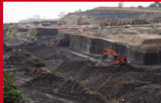
The concrete pouring at the Third Set of Locks will start in the first quarter of 2011.
