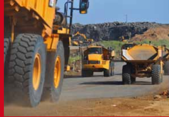
ABOVE: The contractor deployed a significant amount of heavy equipment, which allowed for the excavation of the additional 15,000 cubic metres of material per day.
