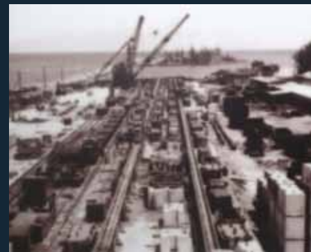
Construction in progress on the Deep Water Harbour in the late 1950s with Pelican Island in the background
